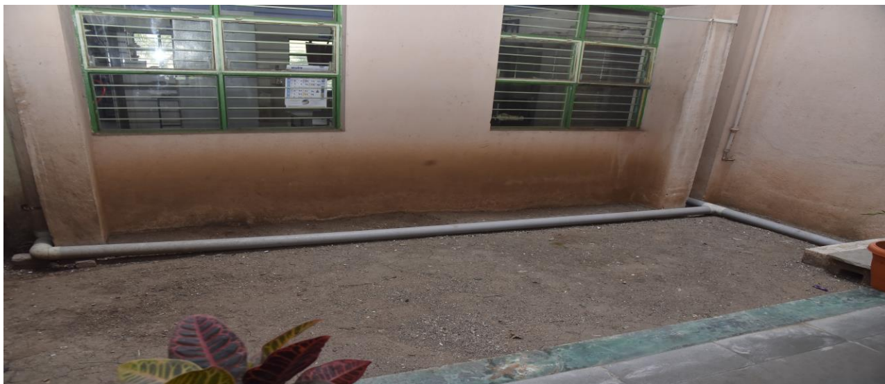
Rain Water harvesting
