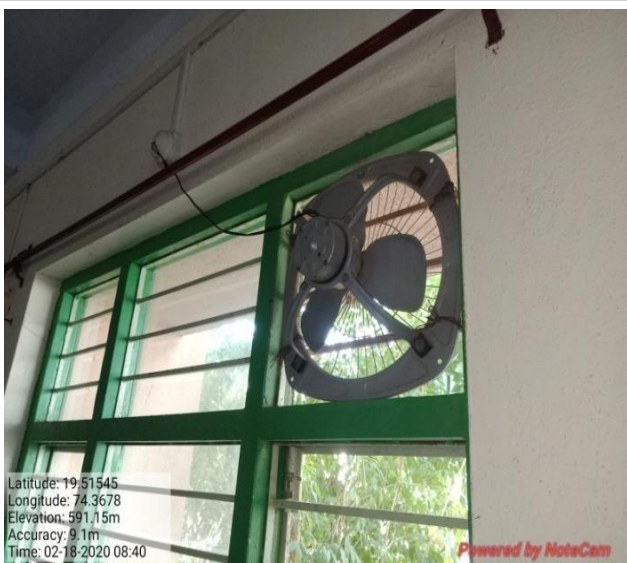
Use of exhaust fan in chemistry laboratory
