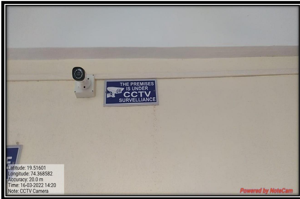
CCTV cameras installed to provide 24/7 surveillance
