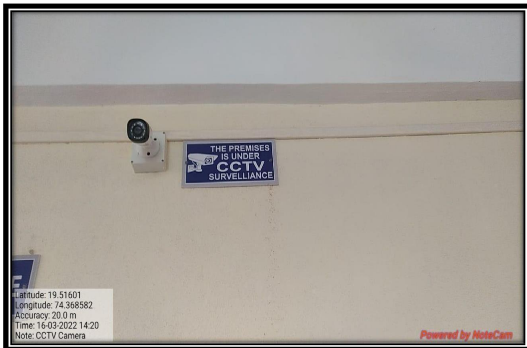
CCTV cameras installed to provide 24/7 surveillance
