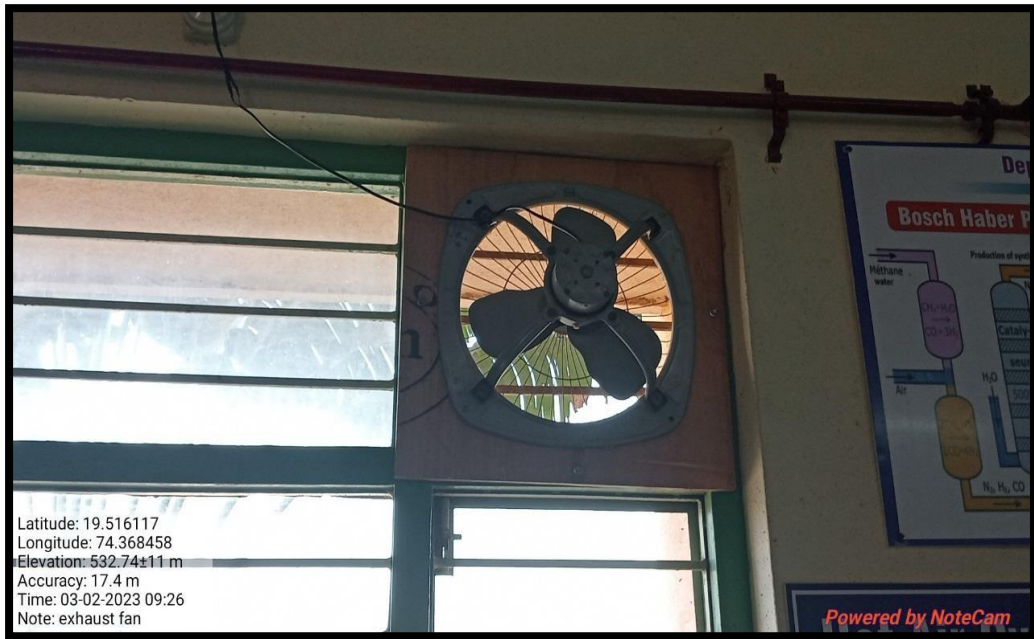
Use of exhaust fan in chemistry laboratory
