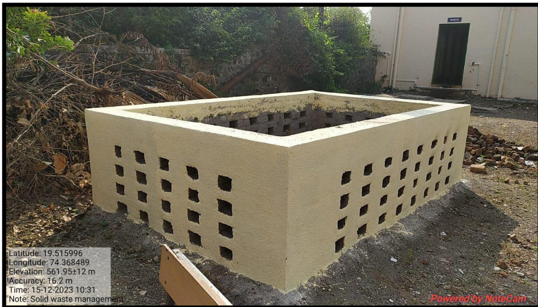
Segregation of Dry Waste
